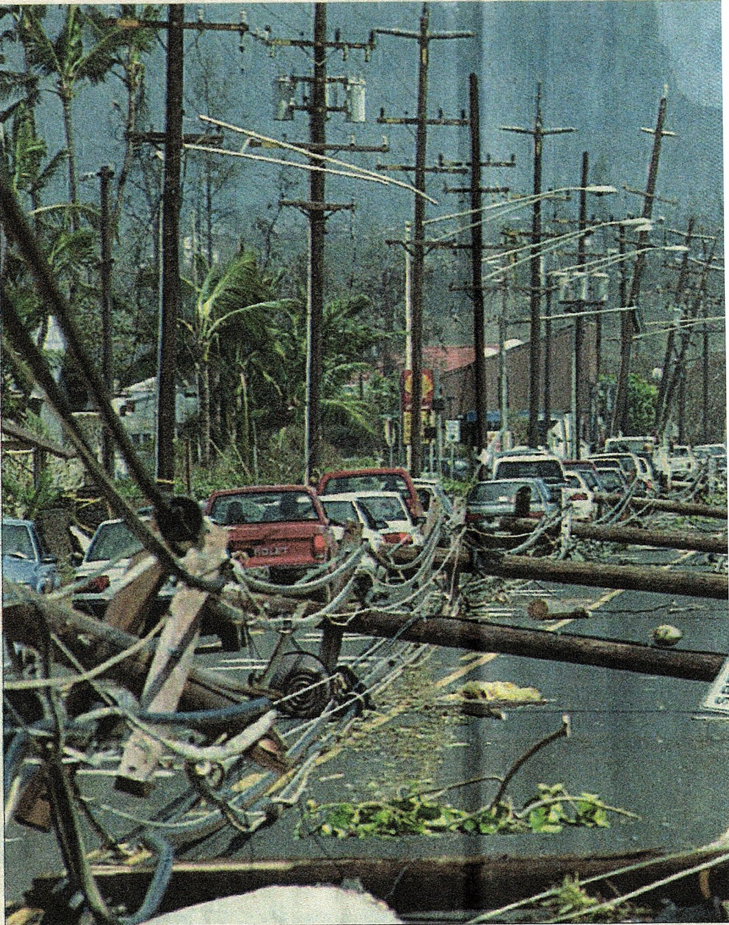
Utility poles fell like dominoes on Kauai after Hurricane Iniki tore through the island in 1992. The destruction
